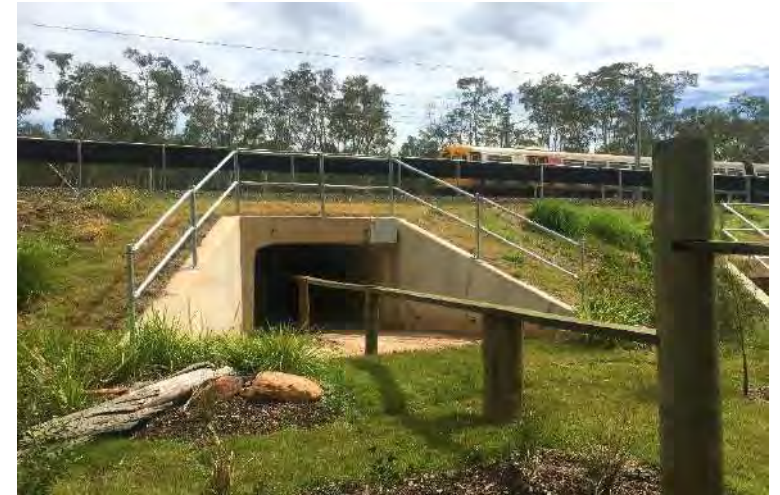
Figure 4.3.12. (photo D de Villiers) A 3.0 m x 3.0 m box culvert provides maximum light penetration and is large enough for fauna furniture to aid movement and predator avoidance.
