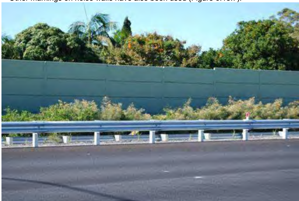
Figure 6.18.6 Solid noise wall barrier (Taylor 2008).
