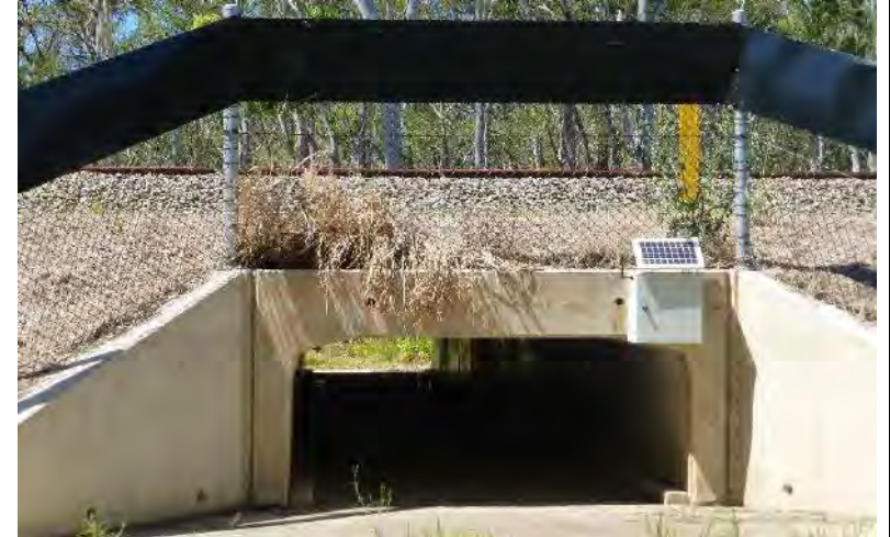
Figure 4.3.14. (photo D de Villiers) Small 900 mm box culverts can still provide movement opportunities for koalas but are too small for the installation of koala furniture and will have reduced natural light penetration.
