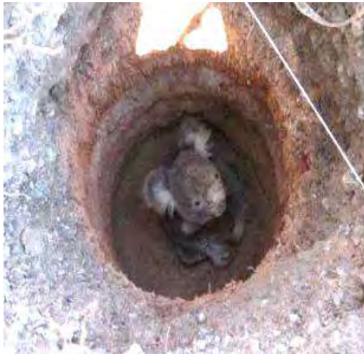
Figure 4.4.8. (photo D de Villiers) Deep post holes for koala proof fencing along a state road upgrade entrapped a koala that could not climb out of the hole.
