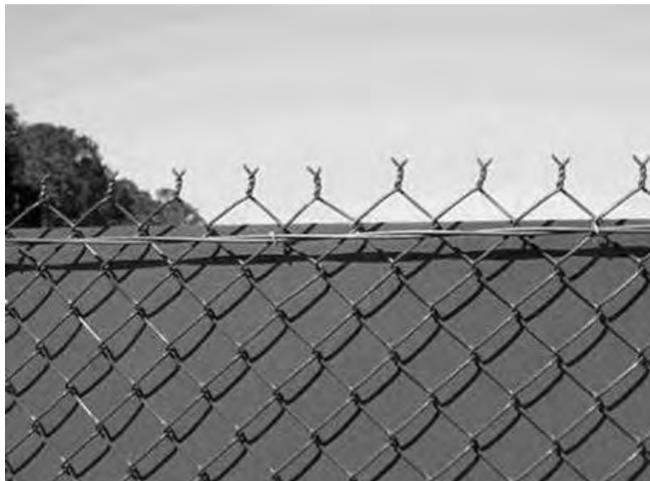
Figure 6.11.2 Incorrectly installed fauna exclusion fencing. For correct installation details refer to Main Roads Standard Drawing 1603.
