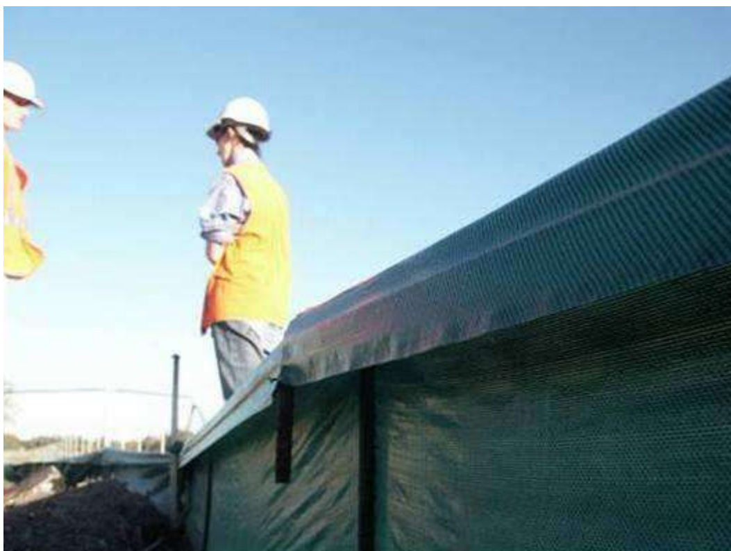
Figure 6.11.10 Temporary frog fence, Tugun Bypass (Robinson-Wolrath 2007).
